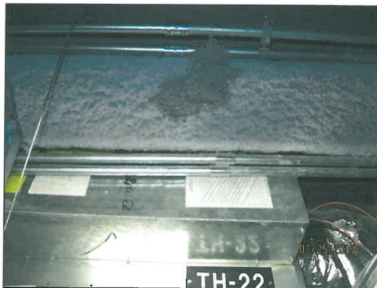
Picture 1. Air terminal unit TH-22 in Room 156 of the Hargray Building.
